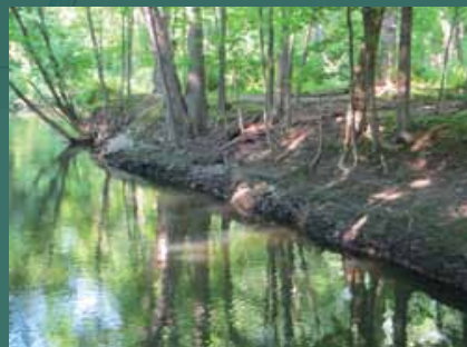
Eroded riverbank, view north from bridge
