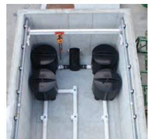
Vault Internal Assembly
