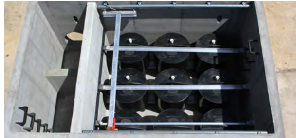
BayFilter Vault Overview
