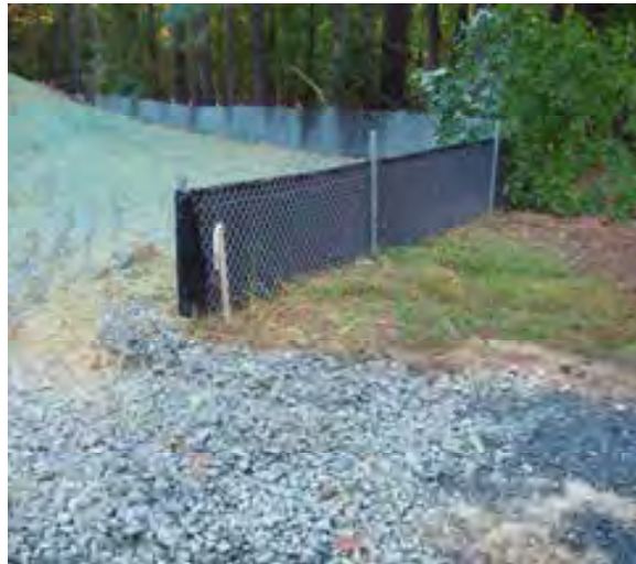
Super Silt Fence
