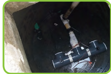
Manifold Tee View of a Cleaned System
