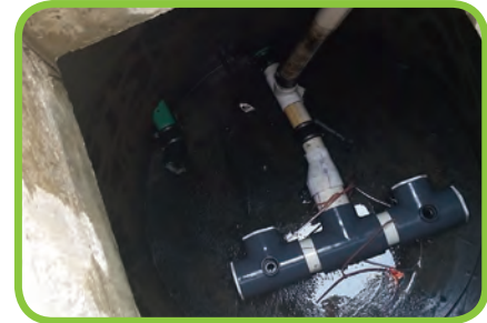
Manifold Tee View of a Cleaned System
